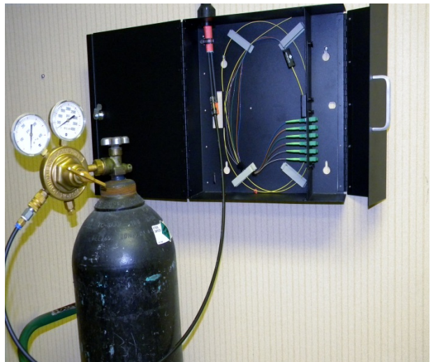
Figure 8 Ready Gas Bottle at Entry Point FTU
